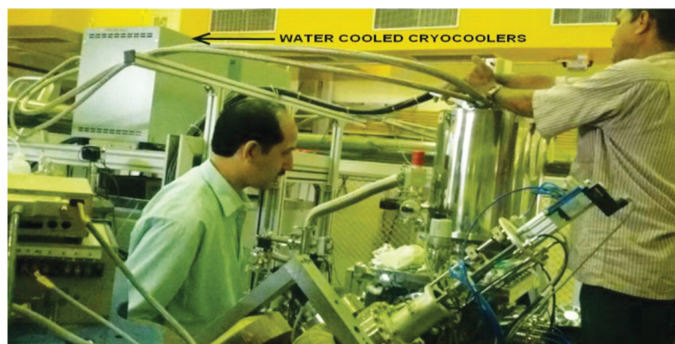
Figure 2.1.6. View of the newly installed water cooled cryo-coolers together with a dedicated water chiller
