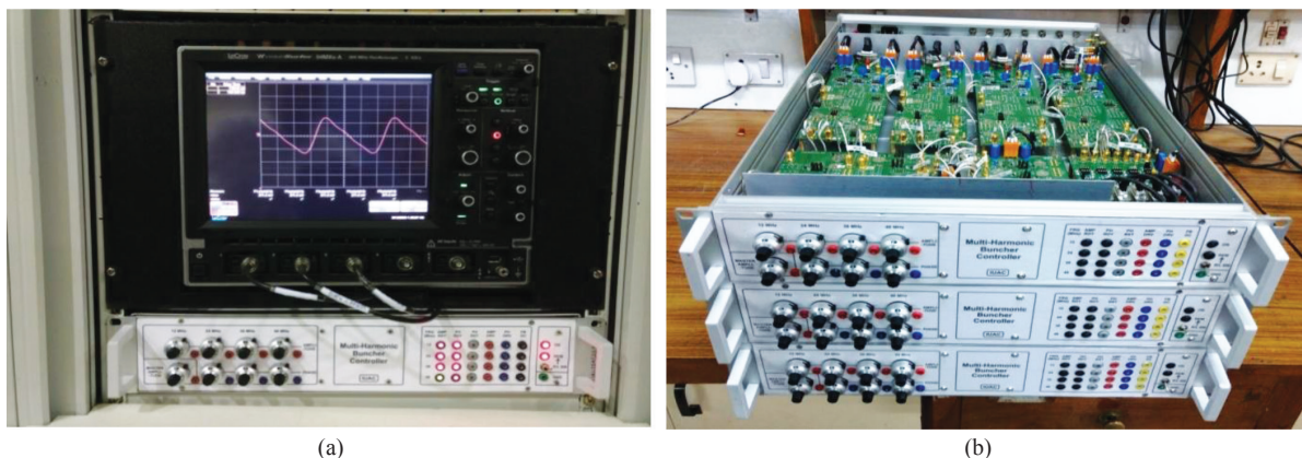
Figure:2.1.23(a) MHB Controller installed in HCI control console (b) the assembled controllers
